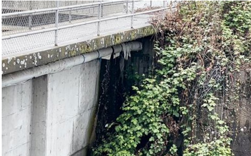
Figure 1. Pipe above South collection channel of East fishway
